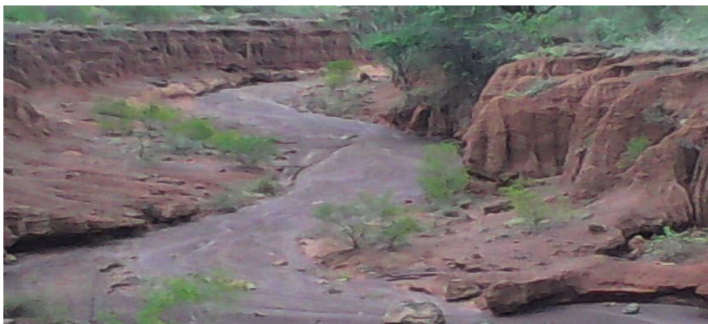
Plate 1: Riverbank erosion along the Lobo river (March, 2013)
