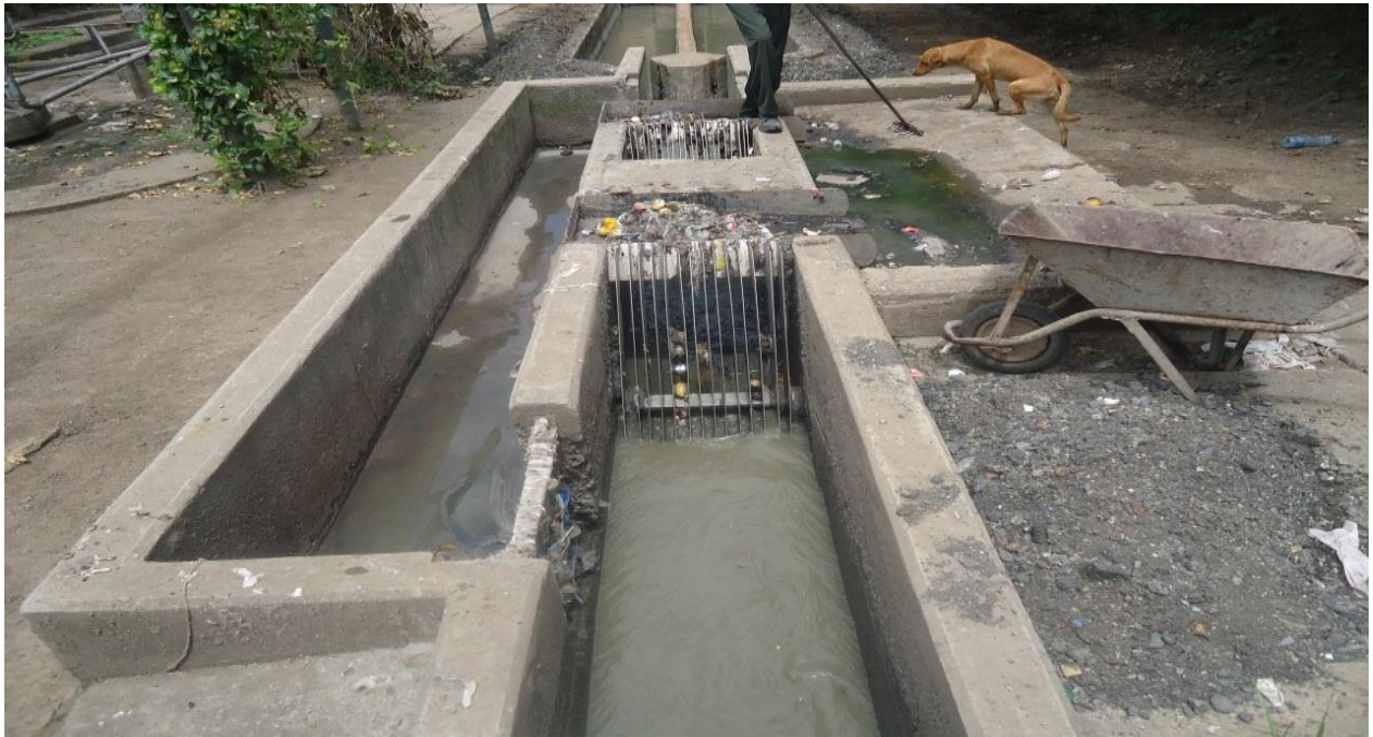
Plate 3.1: In-let of sewage works
