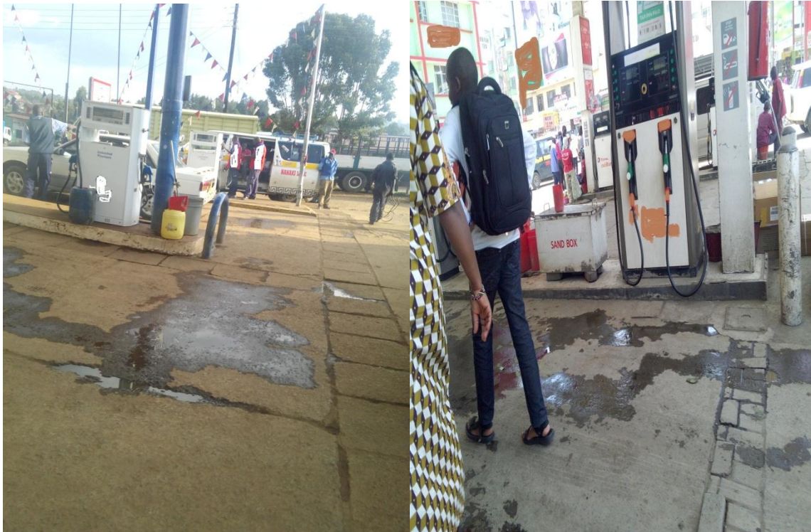
Plate 4.7: Water and Oil Spills at Forecourt Floors of Typical Petrol Stations in Nakuru County
