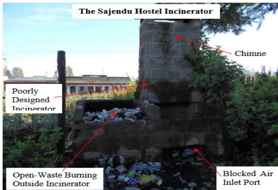
Plate 4.2: Non-performing incinerator at Sajendu Hostel due to poor design.
