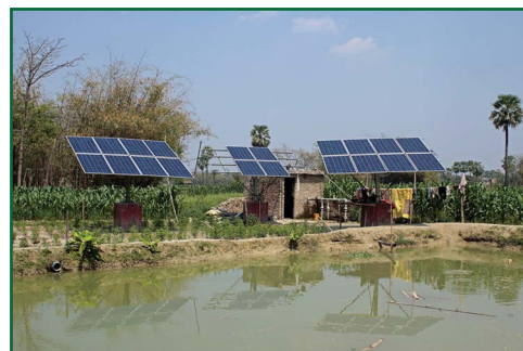
This small dam of rainwater is pumped using solar power to crops during the dry season. Simpler systems are equally beneficial.
