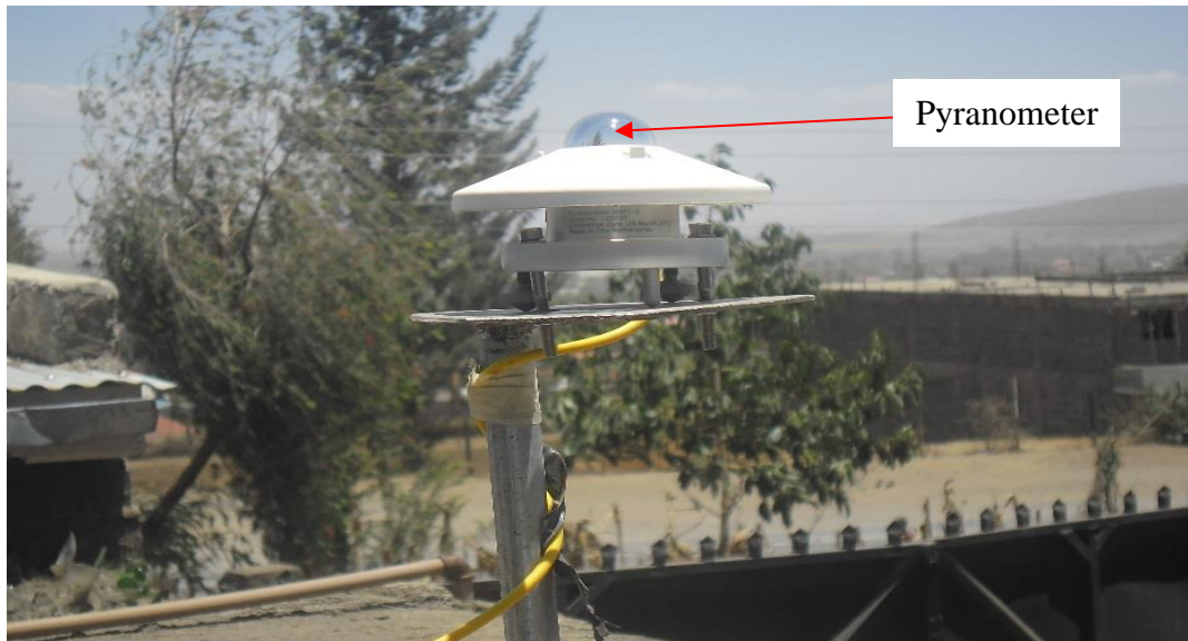
Figure.3.1: Pyranometer mounting and installation
