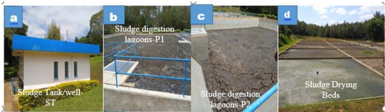
Plate 1: Photographs showing (a) the sludge tank or well, (b) Sludge digestion lagoon-P1 (C) Sludge digestion lagoon-P2 and (d) sludge drying beds located at NYEWASCO-Kangemi WWTP
