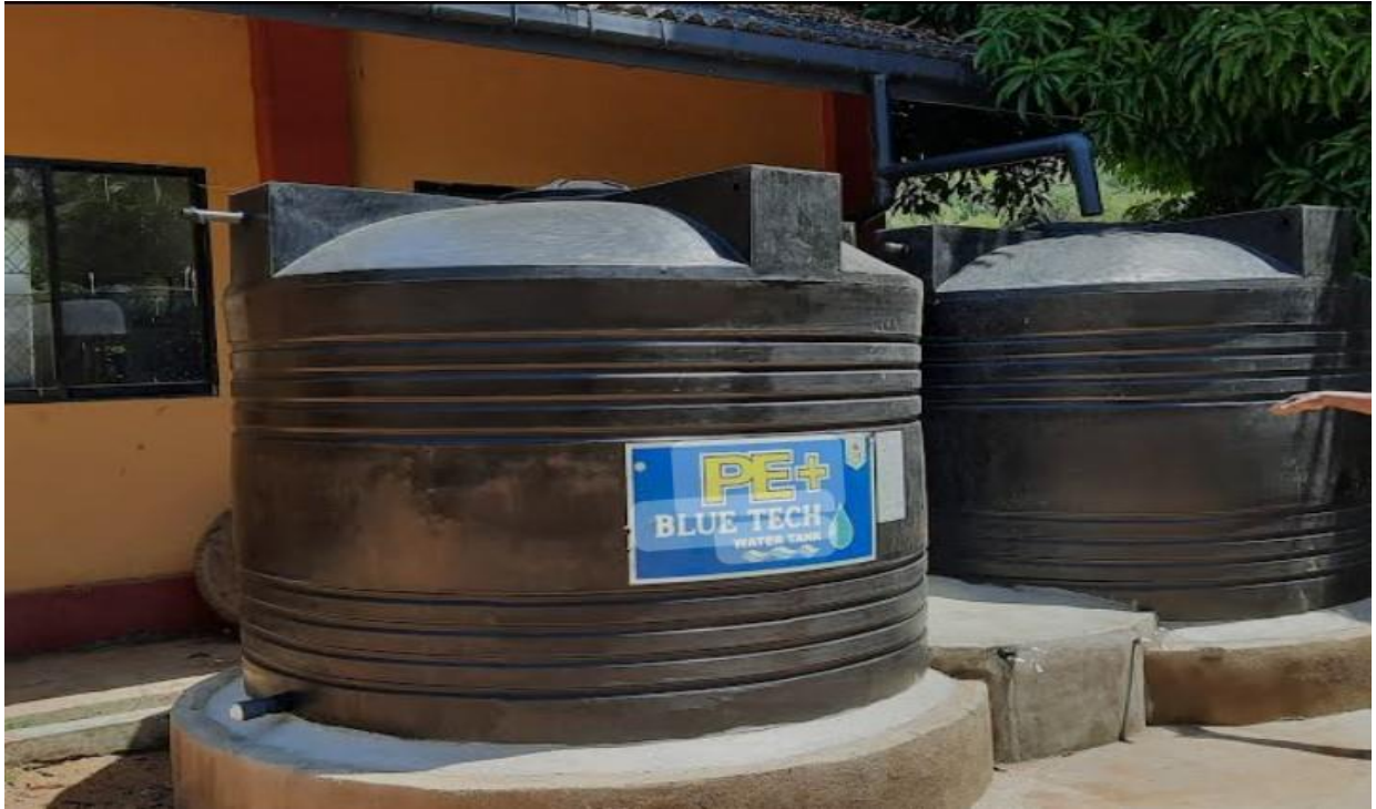
Plate 4.1: A Household in Naka Estate, Nakuru City, Harvesting Rain Water
