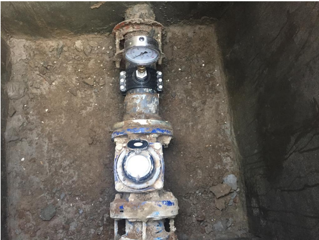
Figure 3.4: Water Meter and Pressure Gauge for Flow and Pressure Measurement respectively
