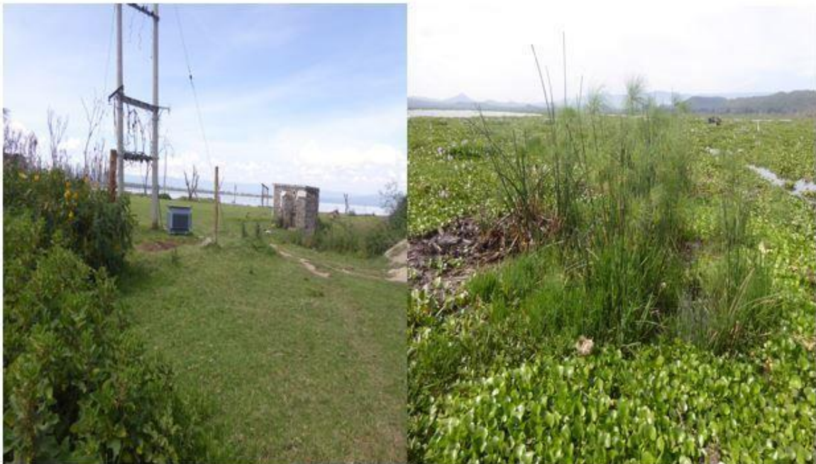
Destroyed horticulture water pump house due to rising water levels in Lake Naivasha
