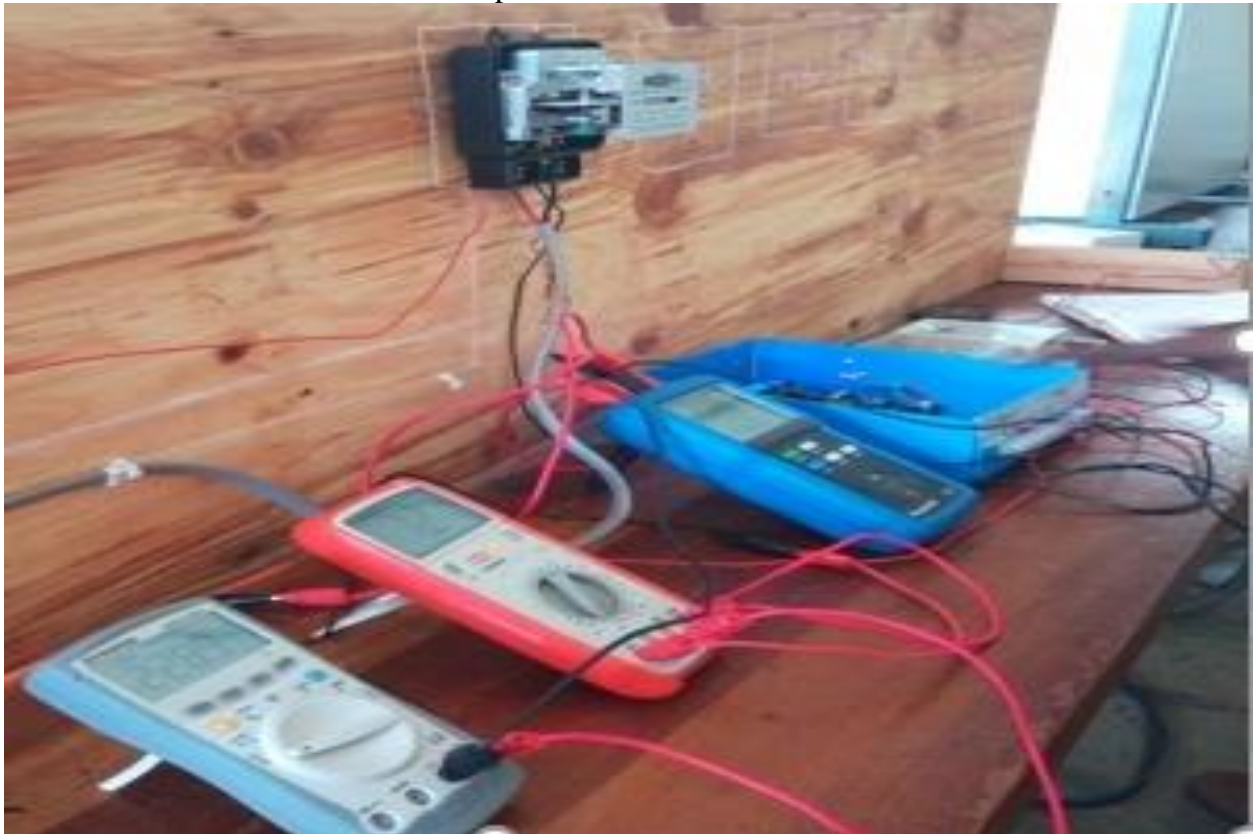
Plate A-3: Vertically-mounted energy meter and other instruments for data collection
