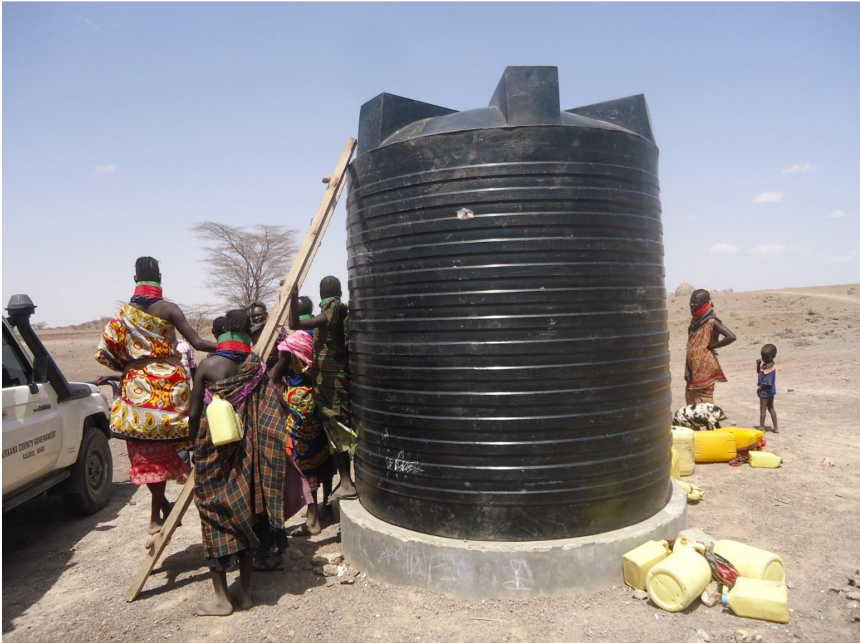
Plate 4.17: A water tank at Nachamae Village, Kapua Location, Turkana Central Sub-County
