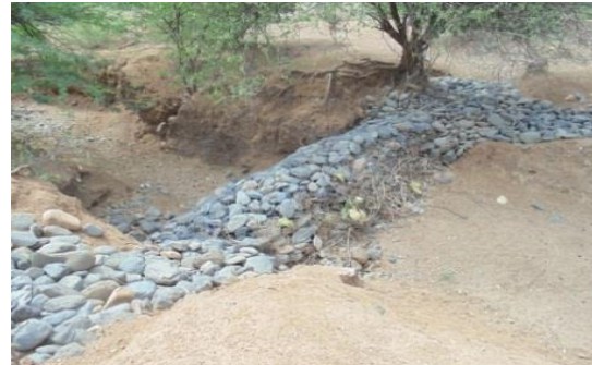
Plate 4.11: Momonyoko (Gabion) at Karwen village, near Chemolingot (Photo by G. Ocarl on 6 th April 2012)
