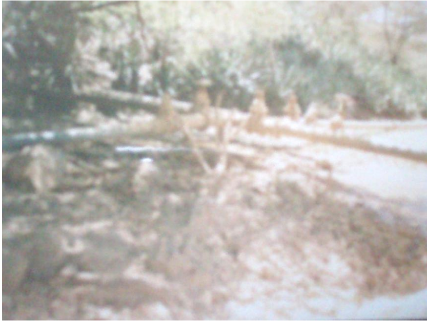
Figure 4.19: Leaking connecting pipes and taps between the sedimentation ponds.
